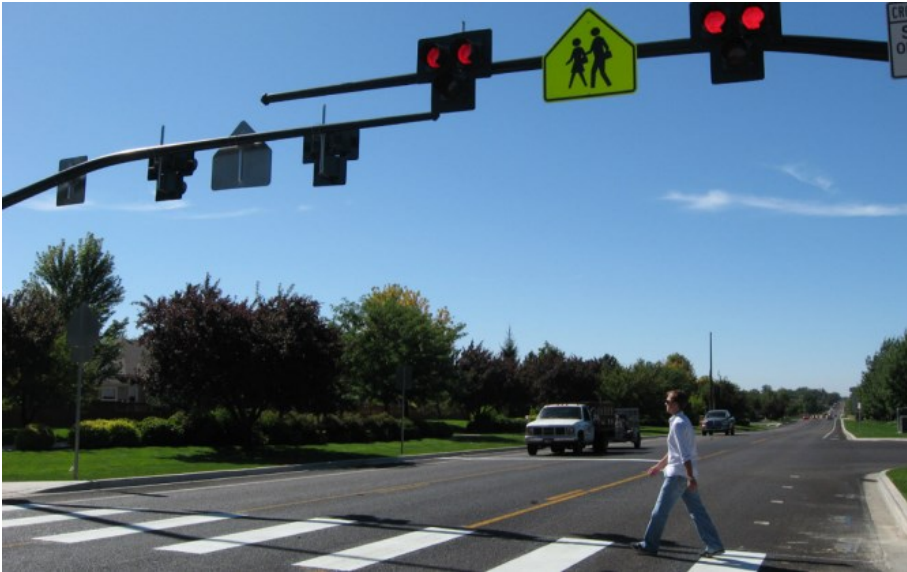
A HAWK Signal alerts motorists to the presence of pedestrians in the crosswalk.
